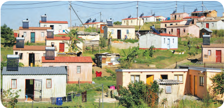
▲ Low cost solar water heaters are installed on Reconstruction and Development Programme housing.
