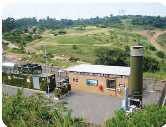
▲ Methane gas from the landfill site is flared off to produce electricity and reduce the carbon footprint of the site
