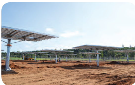
▲ The CPV new Solar Project is the largest installation in South Africa
