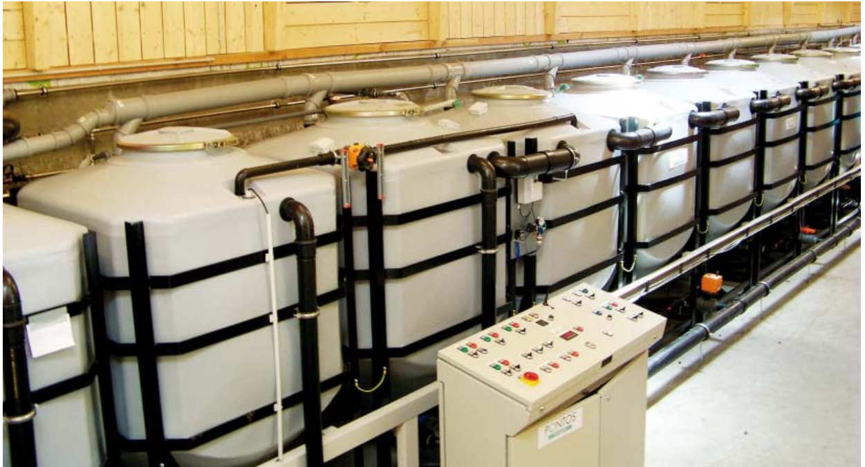
► Figure 2: INTEGRATED WATER CONCEPT IN BLOCK 6 IN THE CENTRE OF BERLIN: GREYWATER RE- CYCLING OF HIGH- LOAD GREYWATER INCLUDING KITCHEN AND WASHING MACHINES (10 m 3 /d; 250 PERS.) THE GREYWATER VESSELS SERVE TO HEAT THE OPERATION ROOM DURING WINTER
