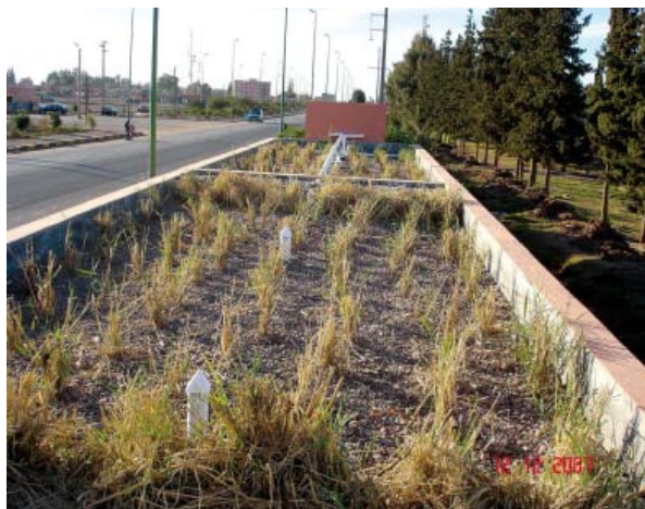
◀◀ Figure 5: INLET OF RAW GREYWATER
