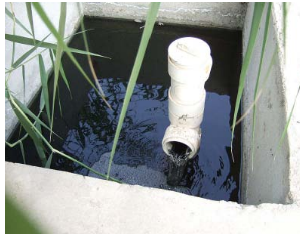
◀ Figure 2: OUTFLOW WELL OF THE TREATED WASTEWATER
