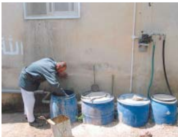
Fig. 1: INSTALLED 4-BARREL GREYWATER TREATMENT SYSTEM
