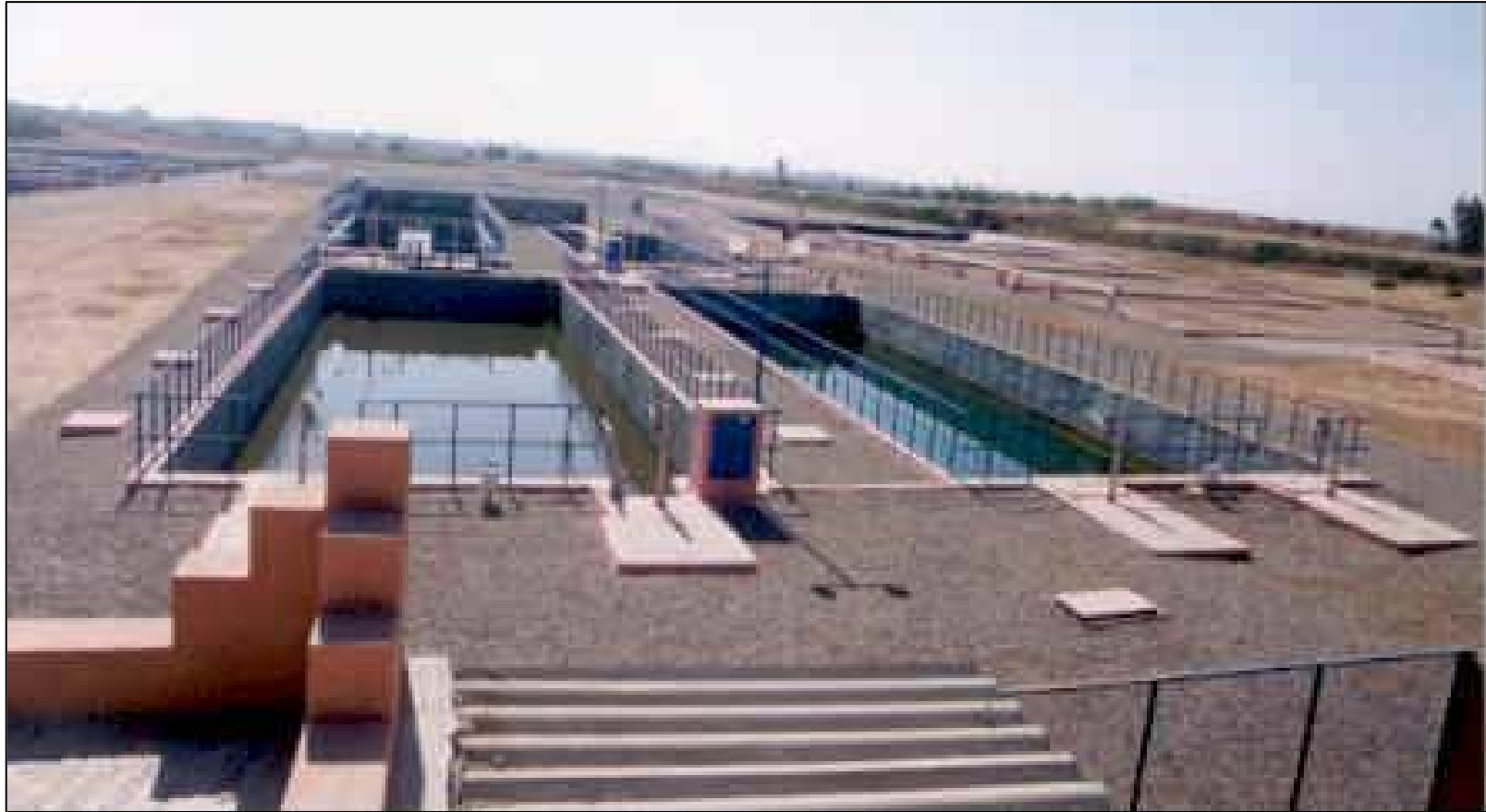
Figure 35: Drarga Treatment Plant (Source: http://www.usaid.gov/ma/successstories/urbansanitation.htm ).
