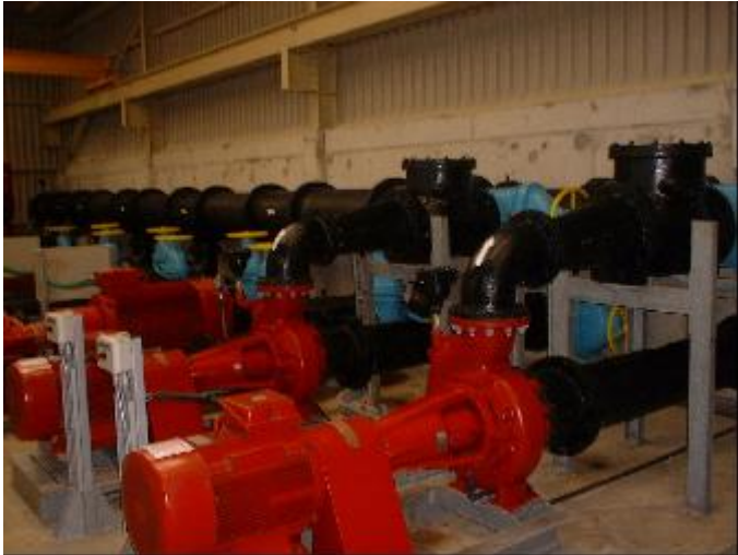
Figure 8. Irrigation Pumping Station.
