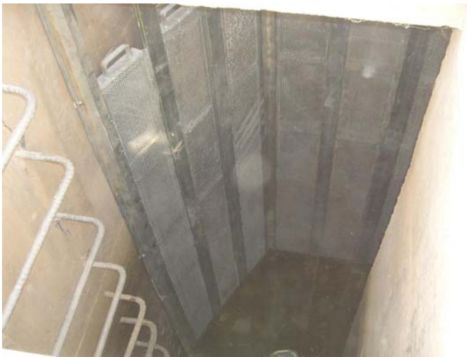
Turn Out 95 (p25) – Detail Grids with mash 10 installed in additional at self cleanning grids for greater protection to the pumping station (extra work contract) King Abdulla Canal – Jordan – August 2008
