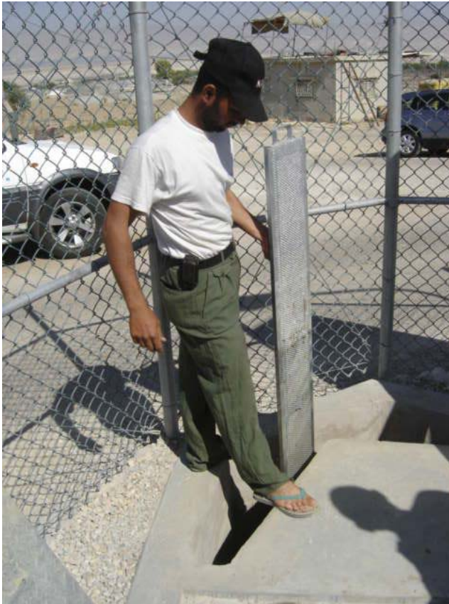
Turn Out 95 (p25) – Detail Grids with mash 10 installed in additional at self cleaning grids Cleaning is done manually ) King Abdulla Canal – Jordan – August 2008
