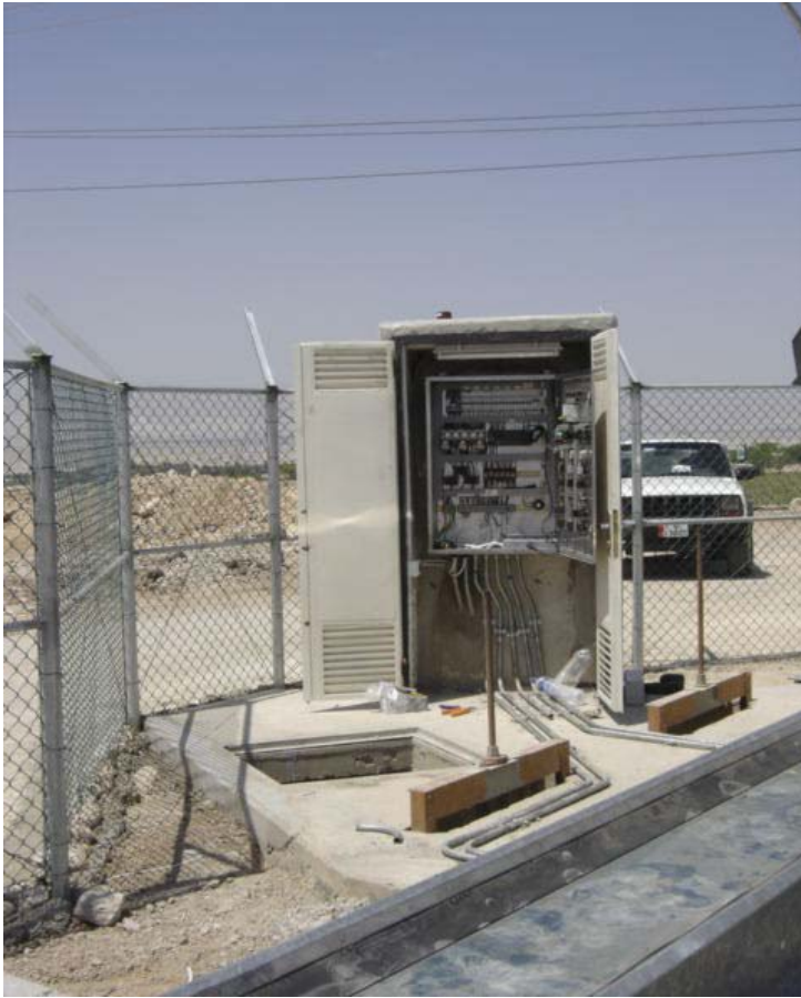
Turn Out 95 (p25) – Detail Control Pannel King Abdulla Canal – Jordan – May 2008
