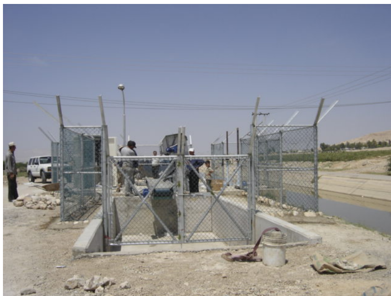
Turn Out 95 (p25) – Detail of ramp garbage container King Abdulla Canal – Jordan – May 2008
