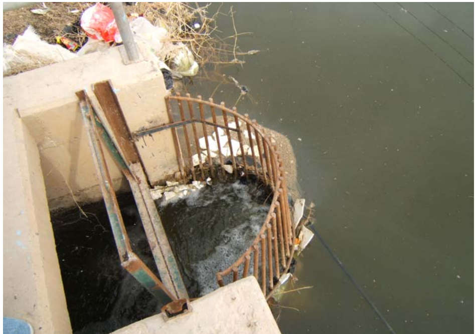
The standard inlet at the TO on the KAC: the quality of water is quite bad and the preliminary filtration clearly unsatisfying.
